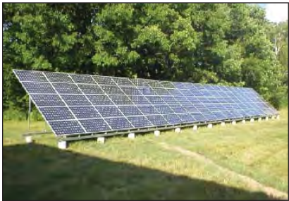
Ground-mounted solar electric array (Source: National Renewable Energy Lab [NREL])
